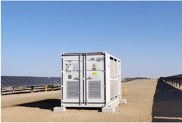
Poland | Solar Noyak Project YBM29-24/2×0.8-6300
